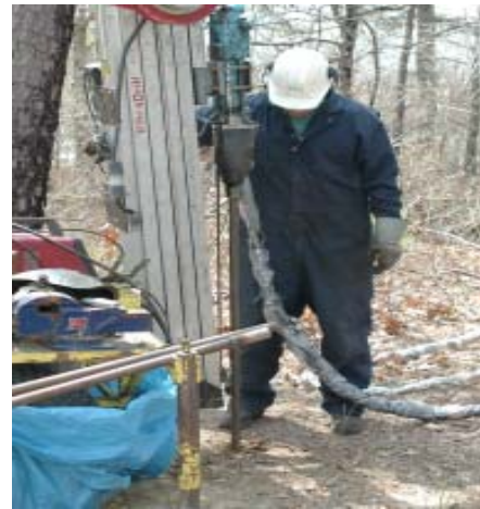
A temporary drive-point is installed in Mashpee Town land, located off Tri-Town Circle.
